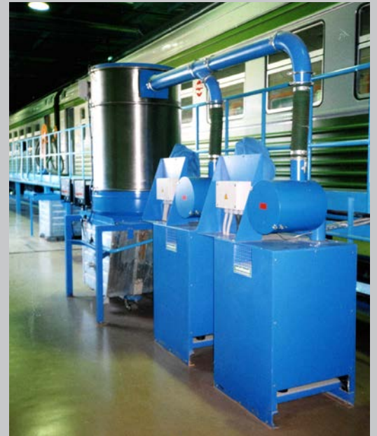
Two parallel vacuum units and a filter hopper. Suction line 200 m in both directions.
