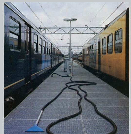
Wet cleaning of railway wagons. The pipework system is mounted under the platform. The suction inlet valves for flexible hoses are positioned under the grate.
